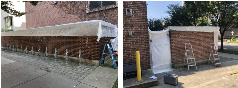
Figure 4. The enclosed area covered in the fire-retardant poly sheeting. In the left image, you can see the sheeting across the enclosed area. In the right image, there was an additional piece of sheeting used to cover the chain-linked gate. The upwind methane analyser (grey box) is placed on the ground next to the door.
