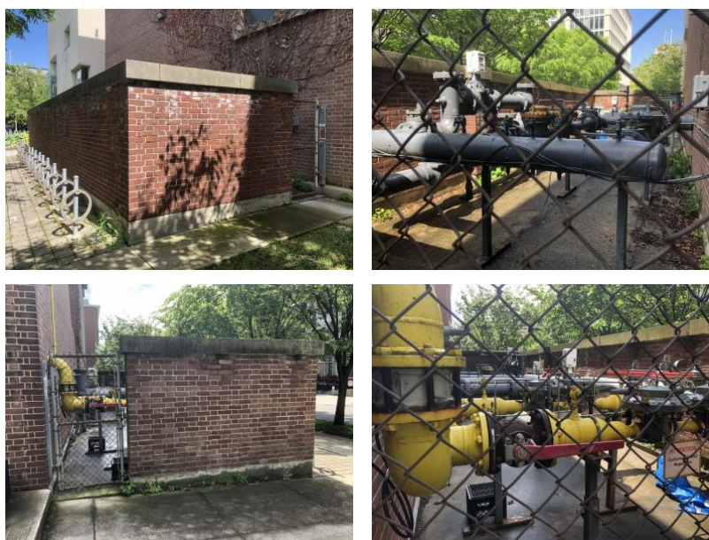
Figure 1. The Central Steam Plant enclosed area. The top-left image shows the north-west corner of the enclosed area. The top-right image shows the view into the enclosed area from the western chain-linked gate. The grey pipes are owned by Enbridge. The bottom-left image shows the enclosed area from the east. The bottom-right image shows the view into the enclosed area from the eastern chain-linked gate.
