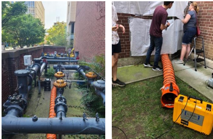
Figure 3. The ducted blower inside the enclosed area next to the audible alarm (running on batteries) (left image), and the blower itself outside the enclosed area with the downwind methane sensor (right image).
